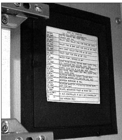
Fuse Panel Label
